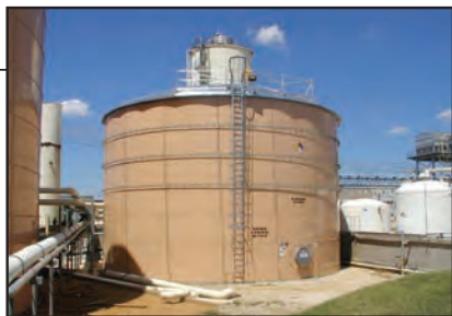
FIGURE 5. Steel bolted tanks with epoxy coatings are commonly used as holding tanks for process water at chemical processing facilities
