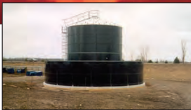
FIGURE 1. Shown here is a glass-fused-to-steel storage tank including a containment tank
