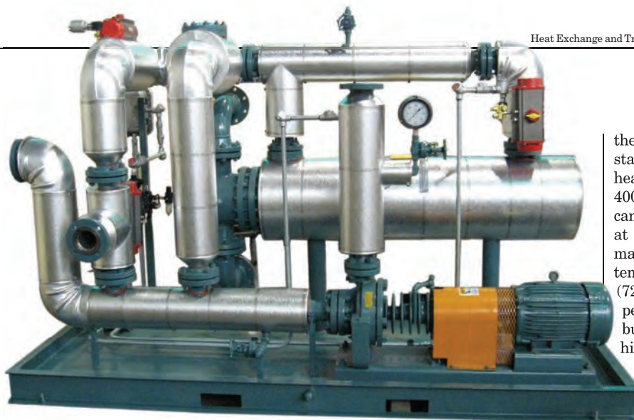
FIGURE 2. This packaged single-fluid system is heated indirectly by direct injection of hot fluid from a central source. The cooling heat exchanger (horizontally mounted behind the pump) cools fluid that is diverted through it by a control valve. The pump maintains alignment by having the casing supported at its centerline. The pump is also air-cooled (note the fins), and the mechanical seal is protected from extreme temperatures by being located at the rear of the pump
