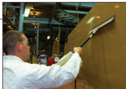
FIGURE 4. An accurate epoxy-coating test includes the use of a high-voltage spark detector, which shows not only the smallest missed spots in the coating, but also spots where the coating does not meet minimum thickness requirements
